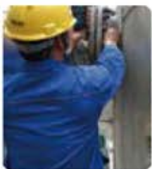
500°C Steam Pipe
