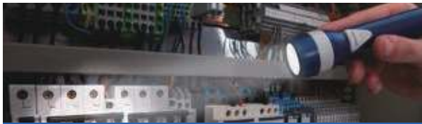
Erroneous circuit-breaker activation
