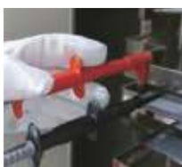
For clamping around the target busbar
