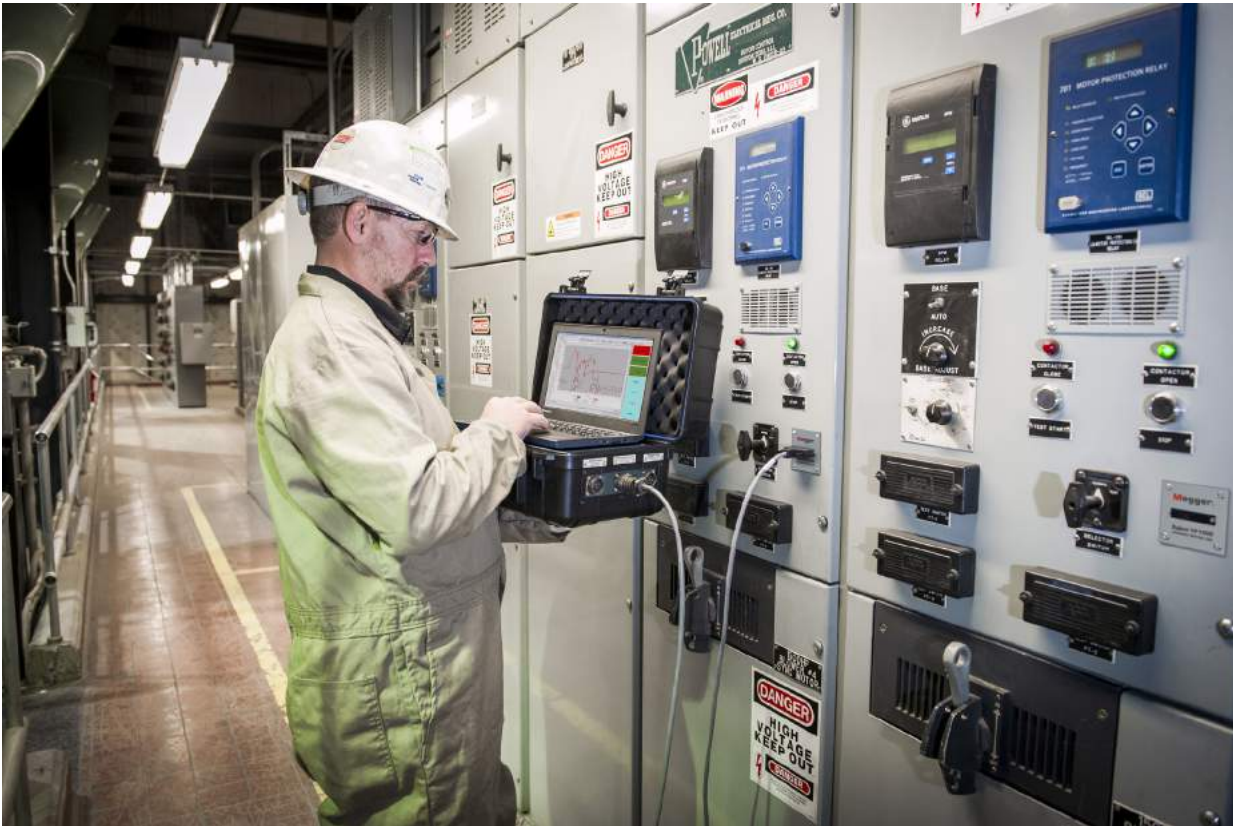
A technician using an EXP4000 analyzer connected to an EP1000 port at an MCC.
