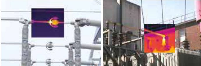
Picture-in-Picture allows a clear overview of these high voltage installations.
