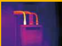
Poor connection and internal damage
