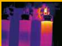
Internal fuse damage
