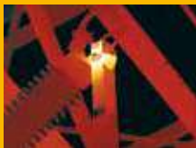
Incorrectly secured connection
