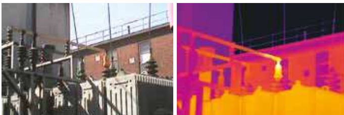
A wide view of a substation can quickly show areas where unwanted high resistance connections exist. No other predictive maintenance technology is as effective for electrical inspections as thermal imaging.
