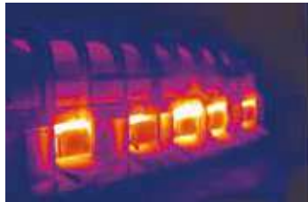
Refractory insulation defect
