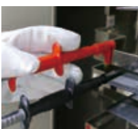
For clamping around the target busbar
